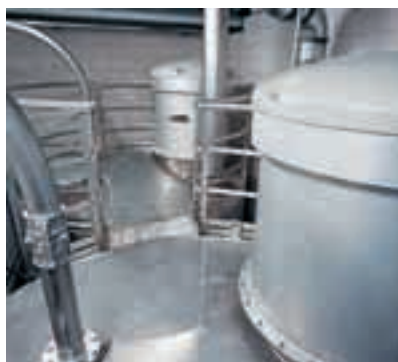
Top of silo with venting filter
