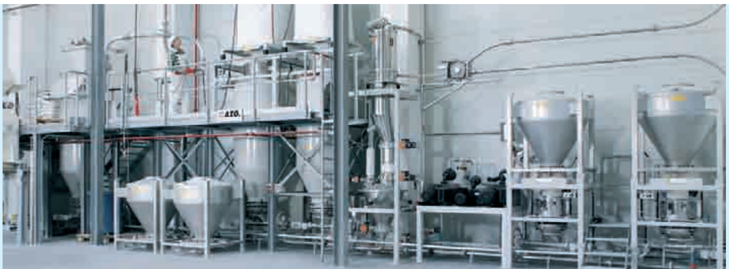
Horizontal material flow through suction weighing systems
