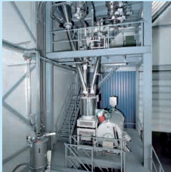
Feeding of heater/cooler mixer
