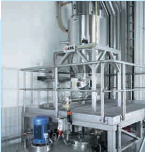
Conveyor scales above stirrer containers in the dairy industry
