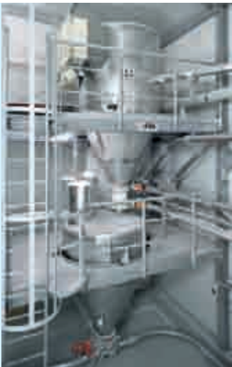
Central weighing station with conveyor scales and buffer container for downstream conveying
