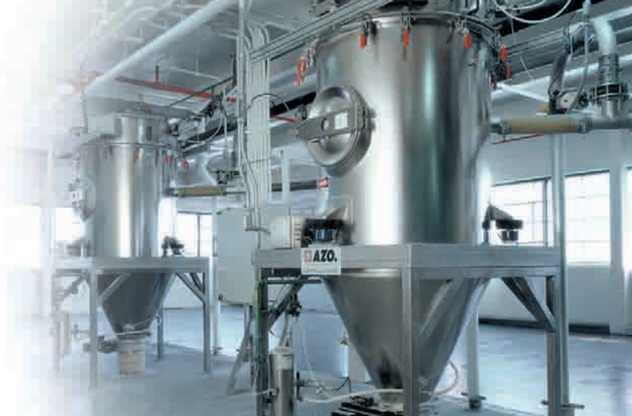
Mixer feeding in the horizontal material flow for convenience foods
