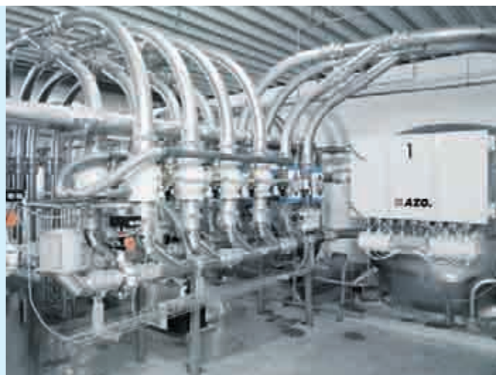
Conveyor scales with multiport valve
